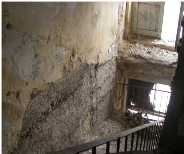
Repairs to the Reception Centre are urgently needed
