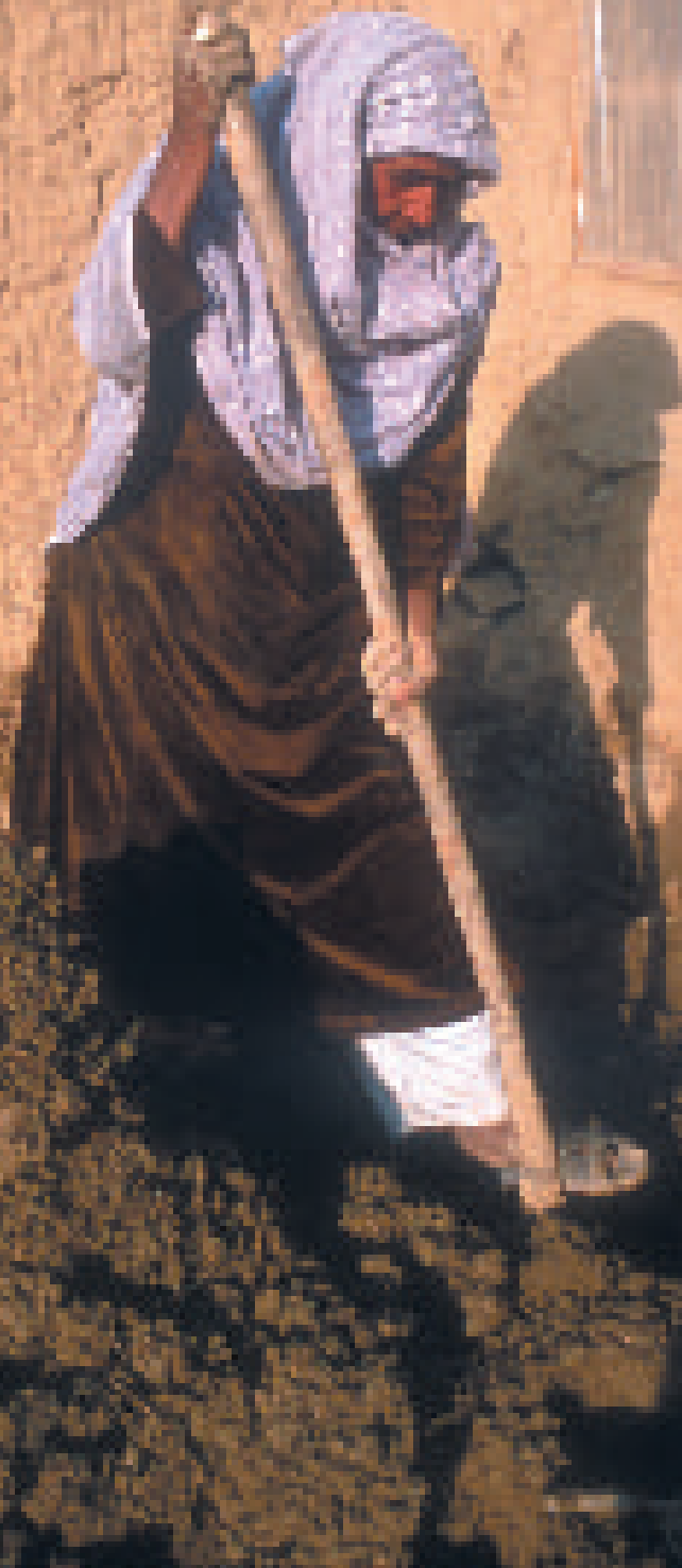
A widow helping her sons to rebuild their house in Kabul. UNHCR/L. Ros
