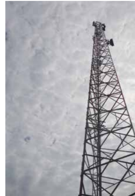
Figure 24: Tanzania/ A new 3G tower built by Vodacom in the middle of the Nyarugusu camp, Tanzania
