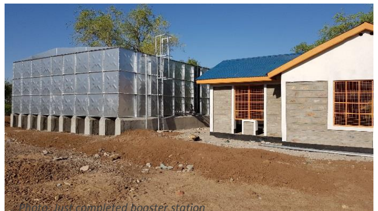
Photo: Just completed booster station
