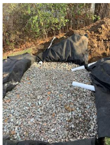
Figure 22: Infiltration trench (Deer Lake Conservancy, n.d.)
