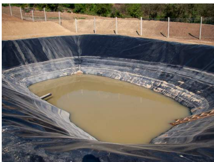
Figure 21: Leachate collection pond with an impermeable liner (credit: iStock joruba)
