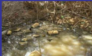
Stagnant water near taps: potential mosquito breeding point
