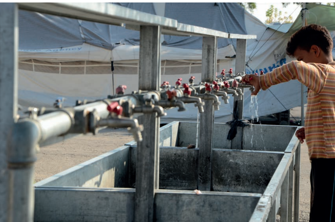
Sanitary and drinking water facilities in Alexandria in a Greek camp, which was established with the help of UNHCR and European Commission funds for Civil Protection and European Humanitarian Aid Operations (ECHO). © UNHCR / ROLAND SCHÖNBAUER
