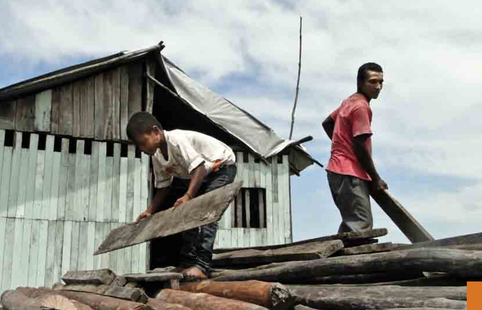
Internally displaced Colombians building homes for themselves in Tumaco, Nariño. (Photo: NRC Colombia, March 2011)
