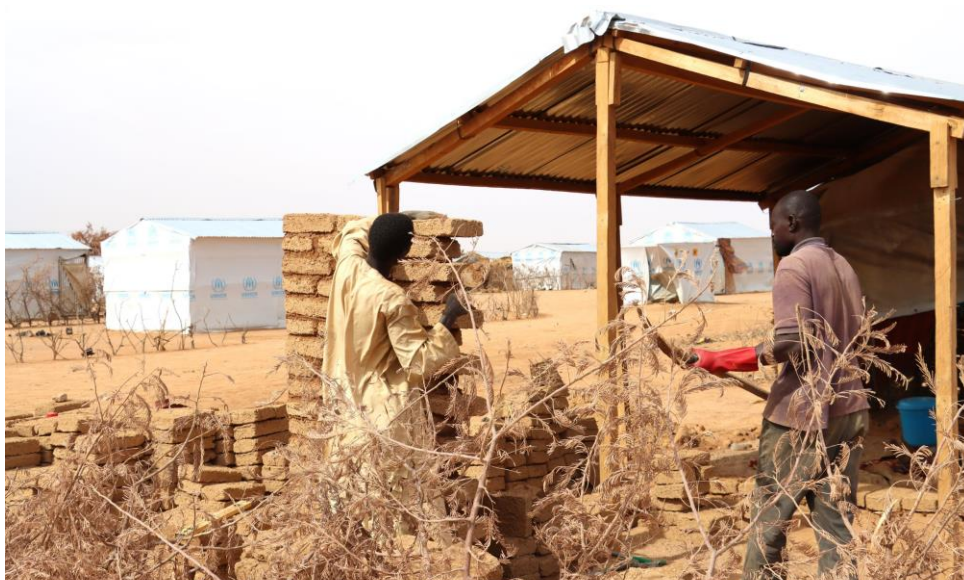
Extension 1 of the Farchana site, Ouaddaï province, welcomes new Sudanese refugees who have found asylum in Chad since 15 April 2023. Ahmat, supported by his friend, decided to transform his mother's shelter into a semi-sustainable mud-brick shelter. © UNHCR/Aristophane Ngargoune
