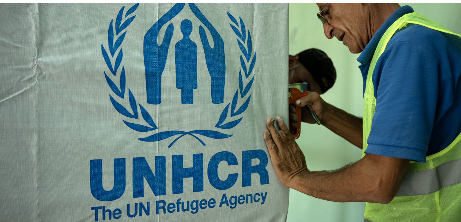
Construction workers assemble partitions, provided by UNHCR, to afford privacy inside classrooms at a Beirut school, where 500 people displaced by the hostilities in Lebanon are living. At least 60 per cent of public schools in Lebanon are now serving as shelters for the displaced. Photo: © UNHCR/Ximena Borrazas
