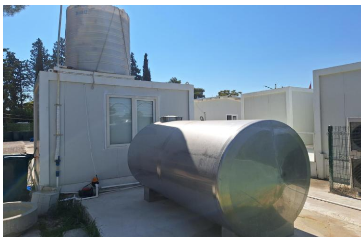
The newly installed water supply system at Karkamış border crossing voluntary return processing centre.
