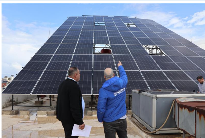
In collaboration with the Ministry of Interior, UNHCR installed a solar power system at the Tartous civil registry office, as part of its growing focus on restoring civil documentation infrastructure. This upgrade ensures uninterrupted services for around 1,700 individuals daily. ©UNHCR/E.Kabbas
