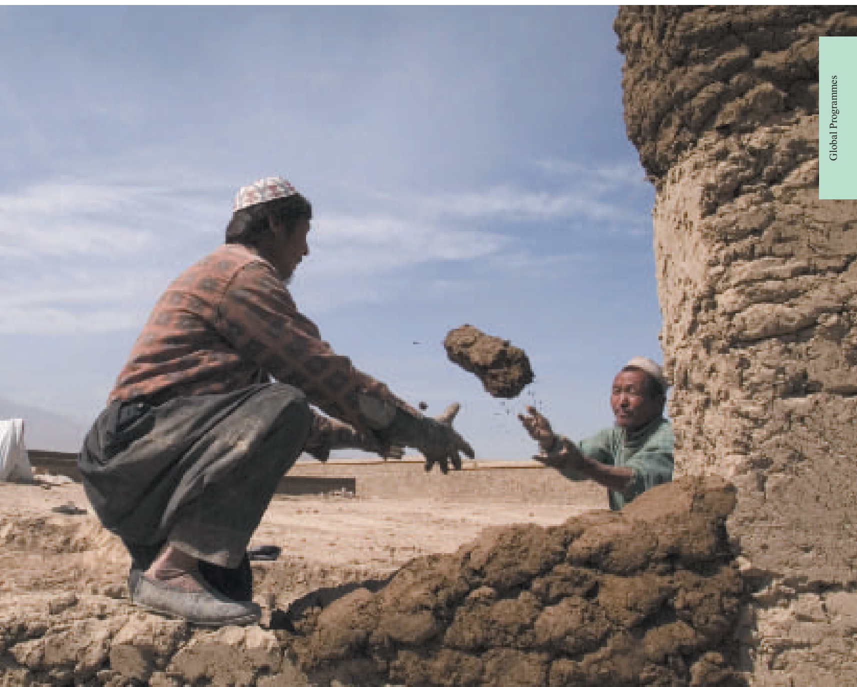
Afghanistan: The Kabul Encashment Centre sees up to 400 families daily who are returning home after having left during the war and the Taliban era. Here, a family is constructing a new home. UNHCR / Lana Slezić / GlobalAware
