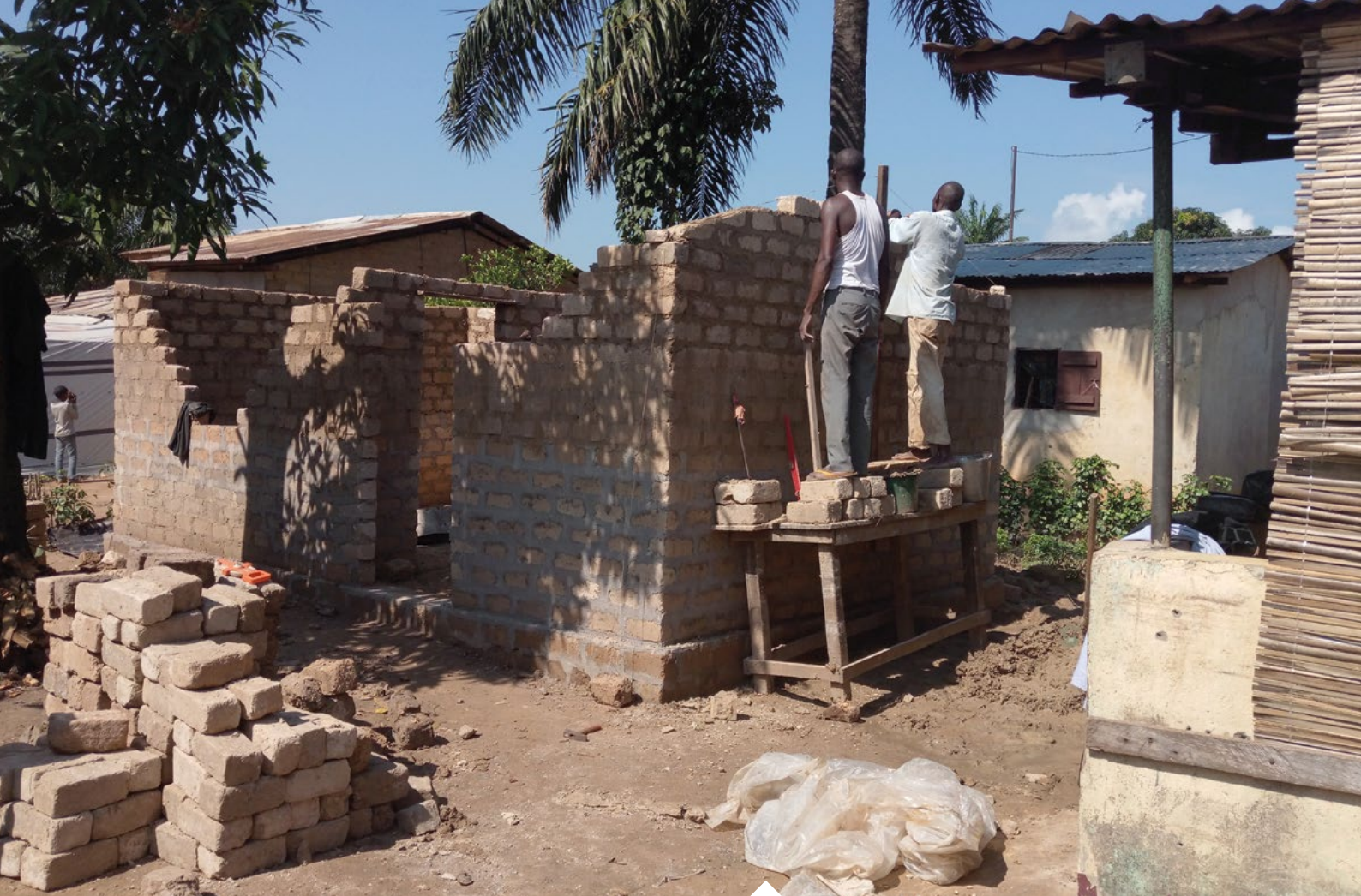
Two men build a house as part of a UNHCR construction project in the Malemaka district of Bangui. © UNHCR/Djerassem Mbaïorem
